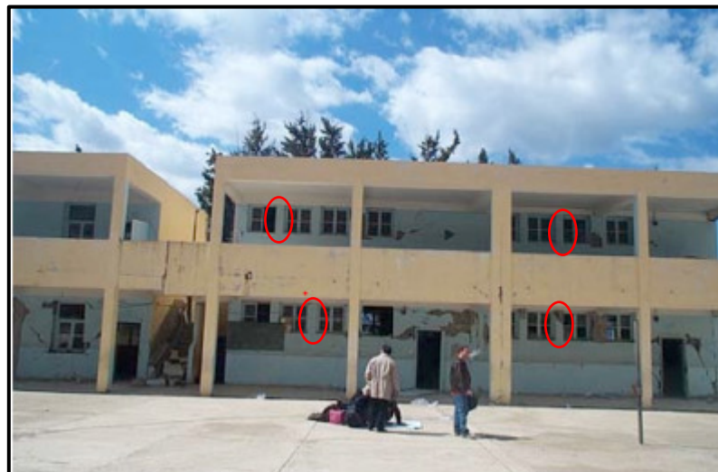
Figure II.8: Short columns effect in Algerian schools.
