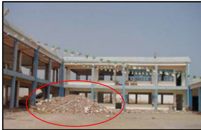
Figure II.6: Masonry infill damage during Boumerdes earthquake.
