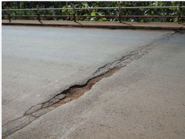
Figure I.18 : fissuration des joints.
