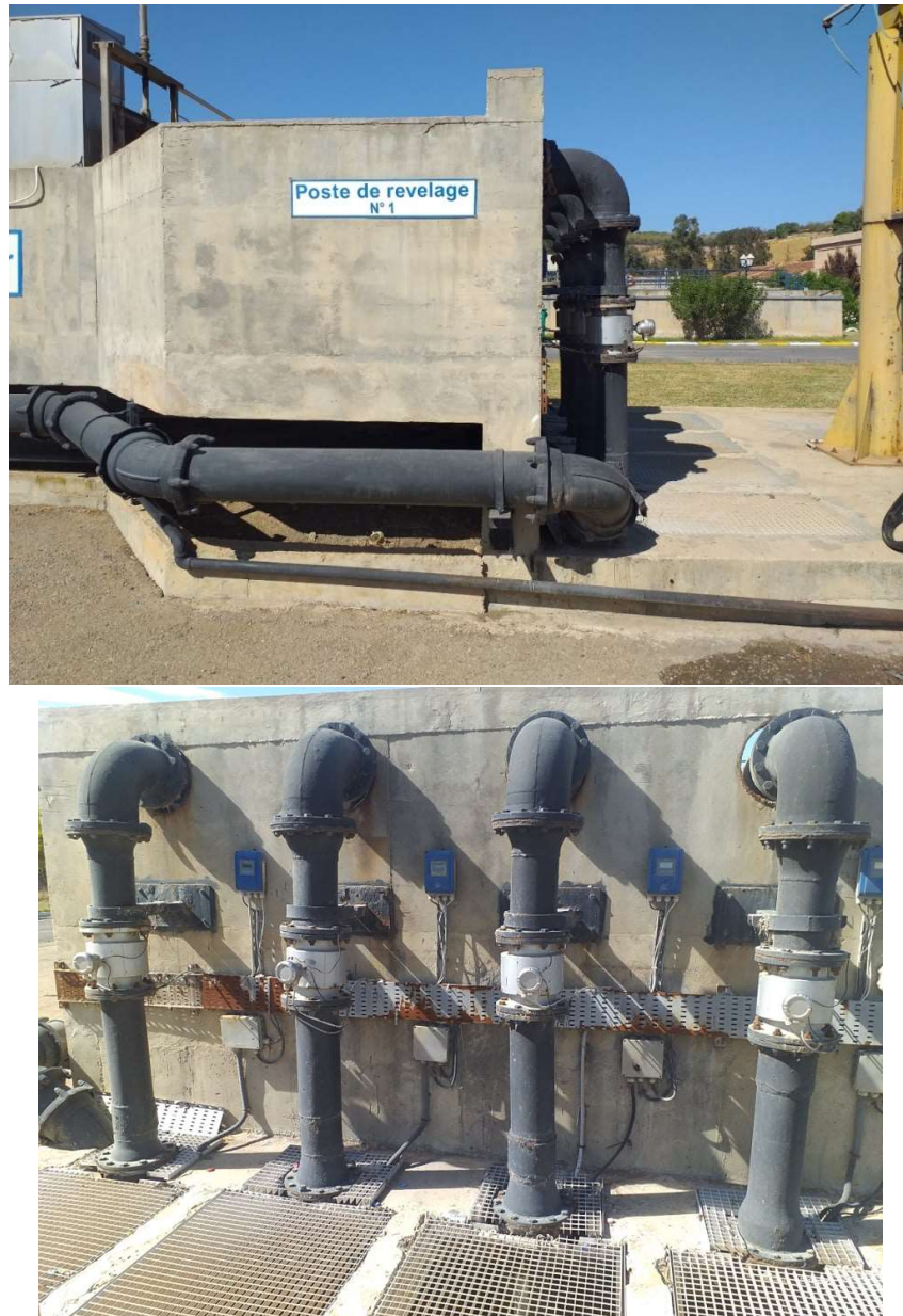
Figure I.6: poste de relevage
