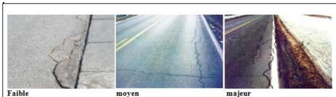
Figure 2.11: Fissures en rive.
