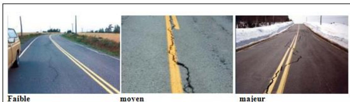
Figure 2.9: Fissures de gel.
