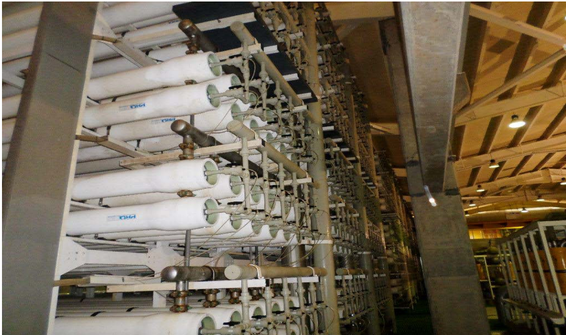
Figure 3.11: Filières d'osmose inverse.
