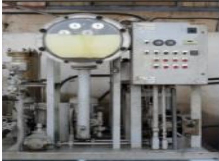
Figure II.5: Station de déshydratation. [33]
