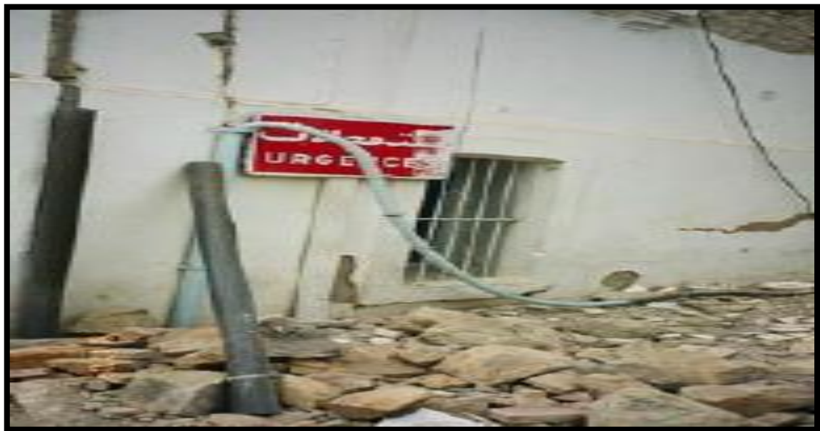
Figure 1. 3: Damage to the emergency wing of Thenia hospital (Achour, 2007).
