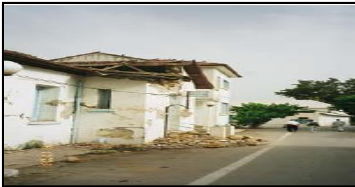
Figure 1. 4: collapse roof of another wing of Thenia hospital (achour,2007).
