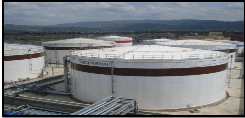
Figure 1.8 : Station fioul combustible
