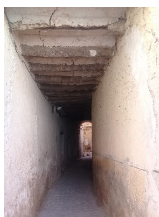
FIGURE : IMPASSE COUVERT A REHABILITE
