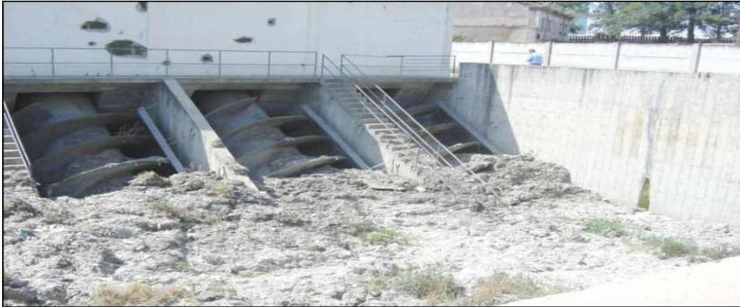
Figure IV.42:Etat de station de relevage SRG 2
