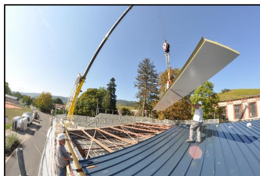
Figure 91 : Couverture panneau sandwich
