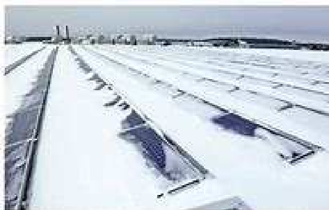
Figure 1.4. Snow on a PV Generator.
