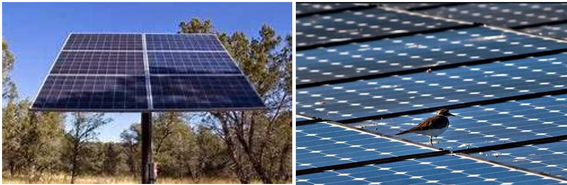
Figure 1.5. Tree leaves and bird droppings on a PV Generator.
