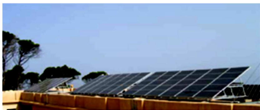
Fig. 2. Roof grid connected PV plant in Algiers, Algeria.
