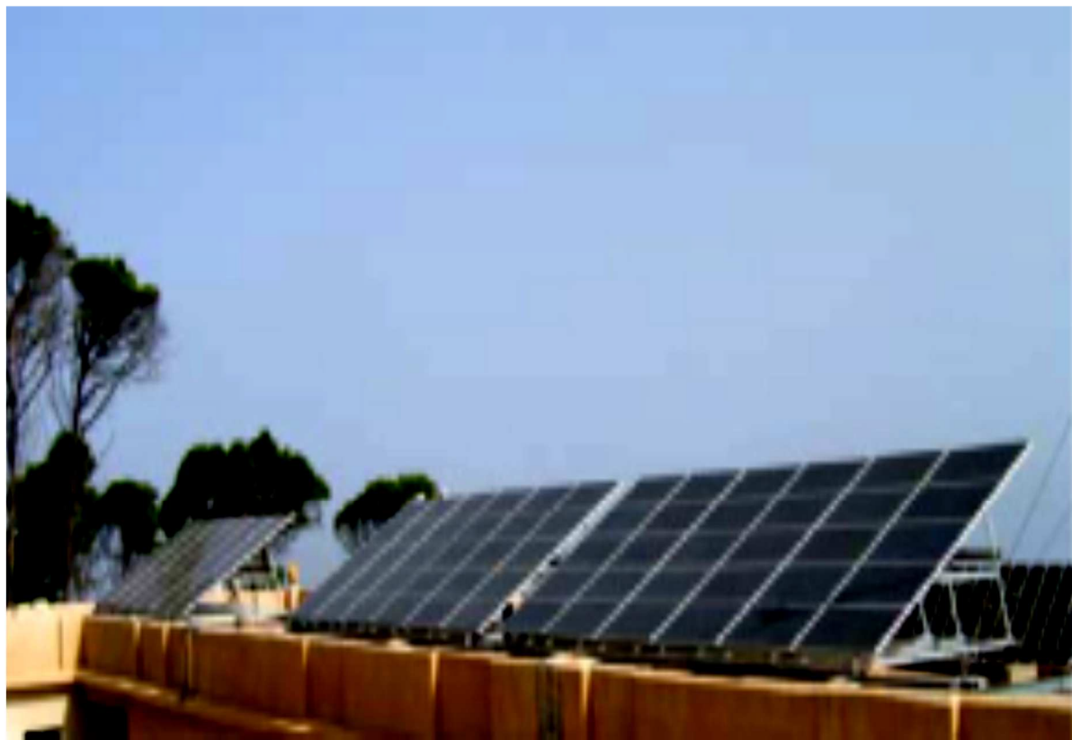
Figure 2.2. Roof grid connected PV plant in Algiers, Algeria.
