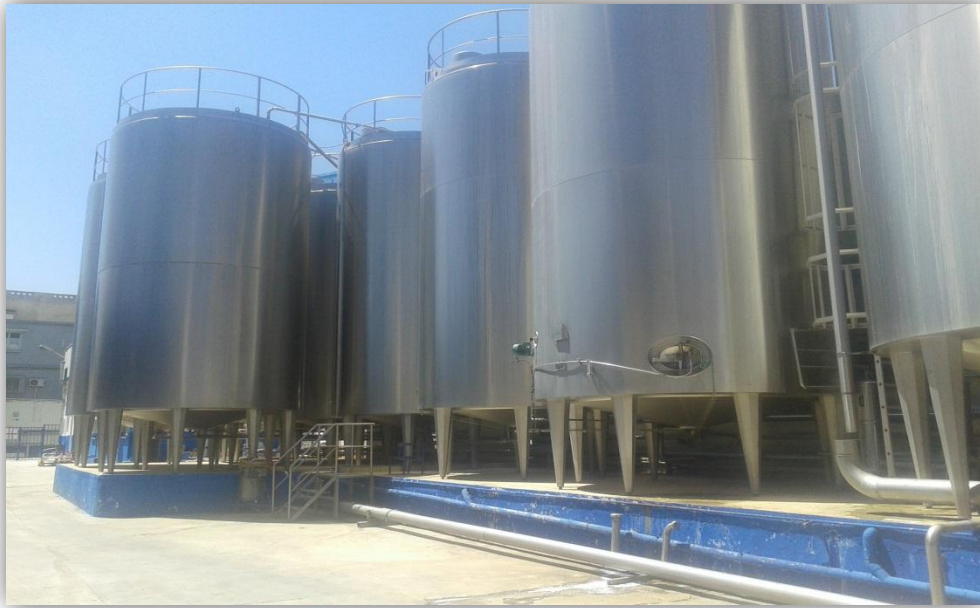
Figure 2.17 : Tanks de stockage.
