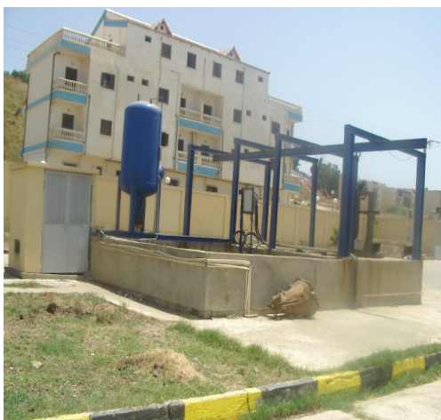
SR2 station de relevage Corso
