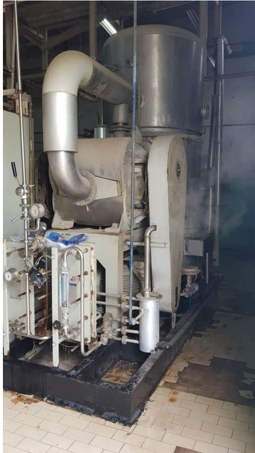
Figure 41 : un distillateur a thermo-compression de la station SMP.
