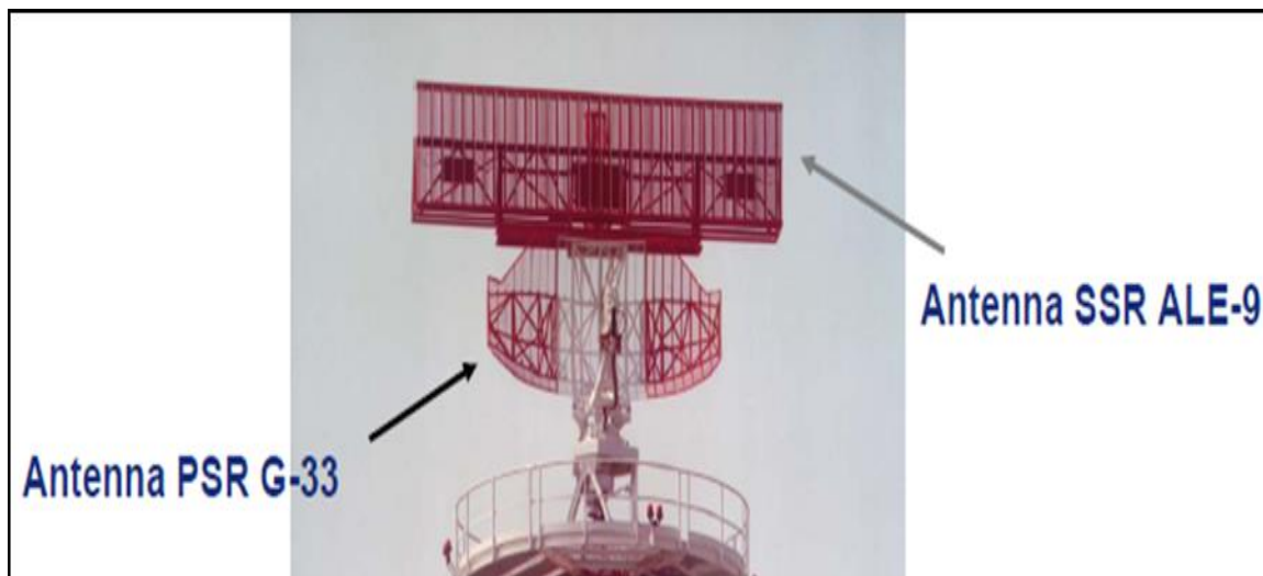
Figure II.2: Antennes radar primaire et secondaire Co-implanter
