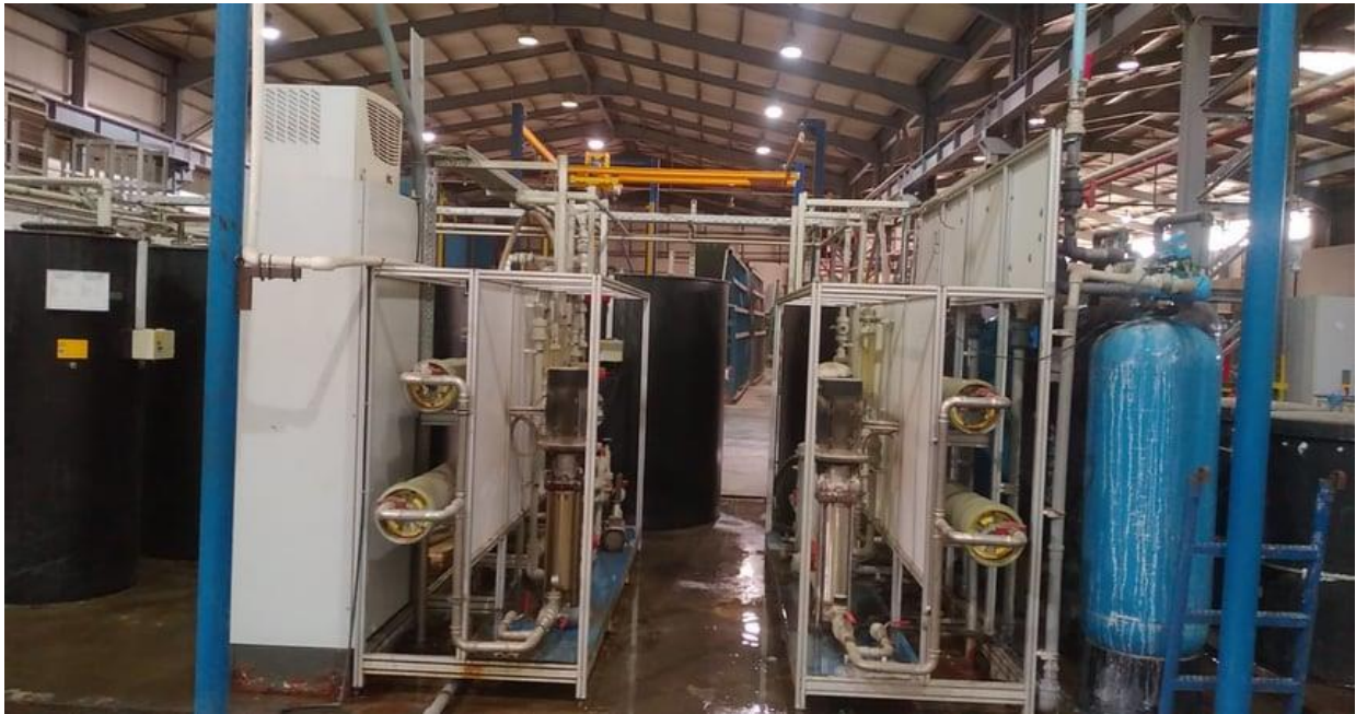
Figure II.1: station traitement d'eau
