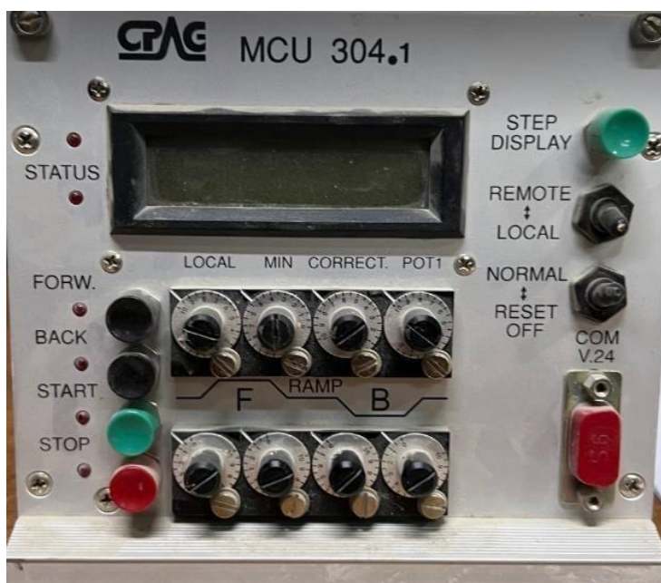
Figure I.14- local commande box (LCB)
