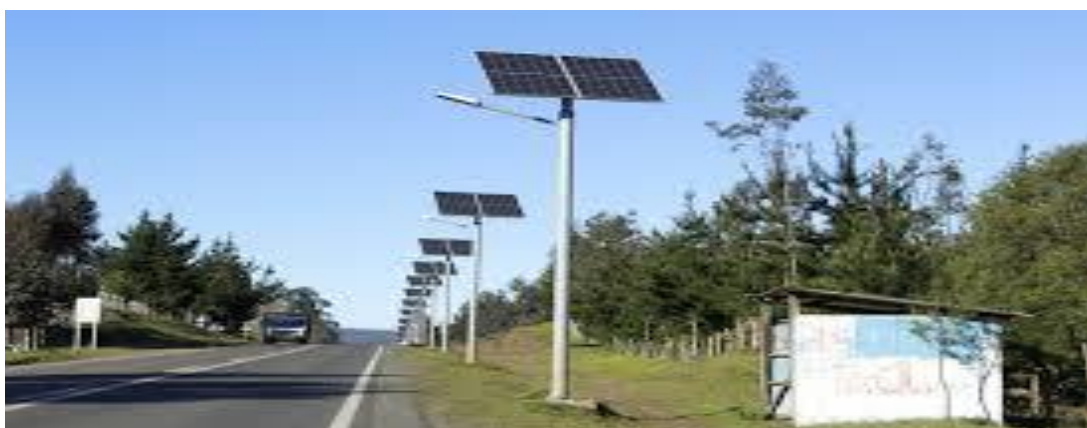
Figure II. 1: Eclairage public solaire
