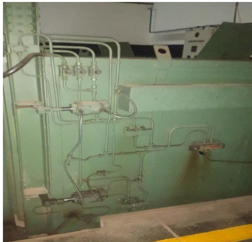
Figure III.7 : Four de stabilisation
