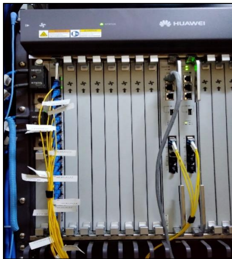
Figure II-14 Optical Line Terminal (OLT).
