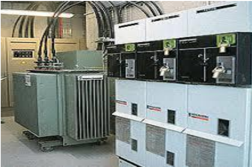
Figure II.5. Poste HTA/BT (DP).
