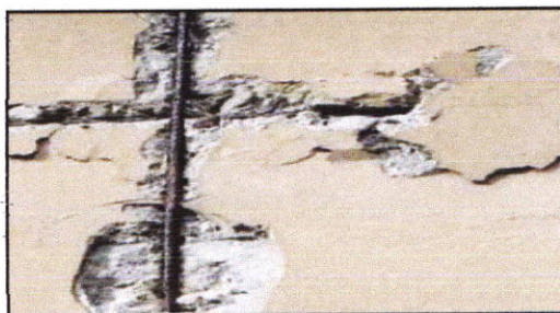
Figure 41. La corrosion source : www.wikipedia.com
