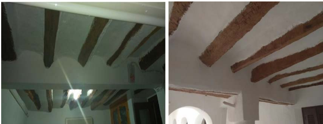
Figure II.7 Photos showing roof of palm tree trunks and vaults in the room of the case study [15].
