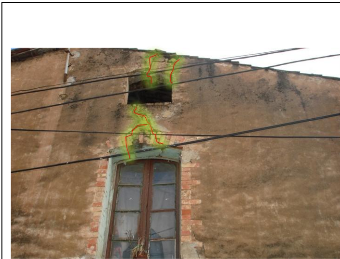
Fig.98 Cas de fissuration
