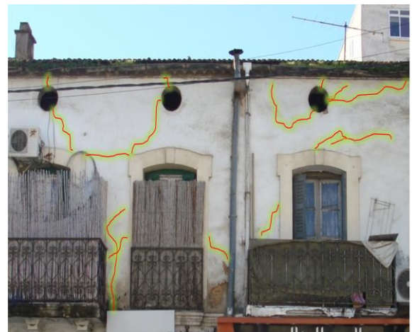
Fig.99 Cas de fissuration
