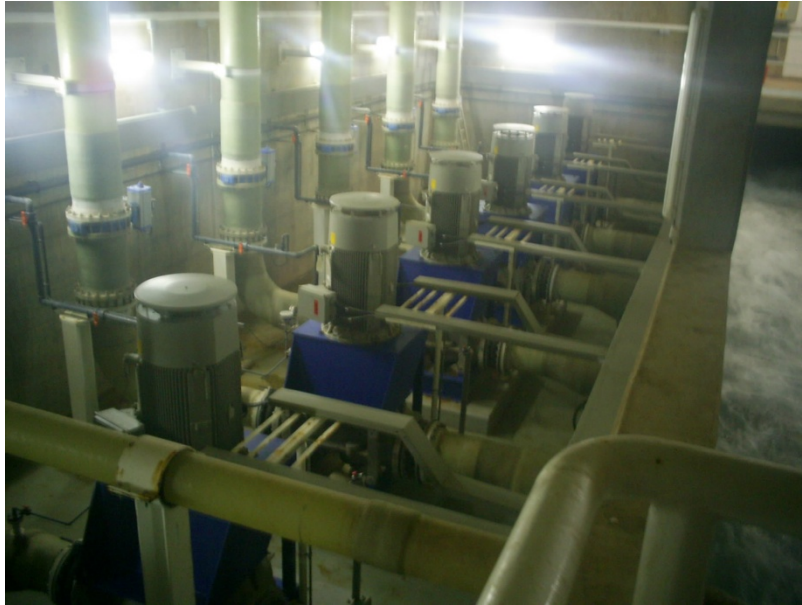
Figure V-5 : Station de pompage, [ source: KHATEB.M].
