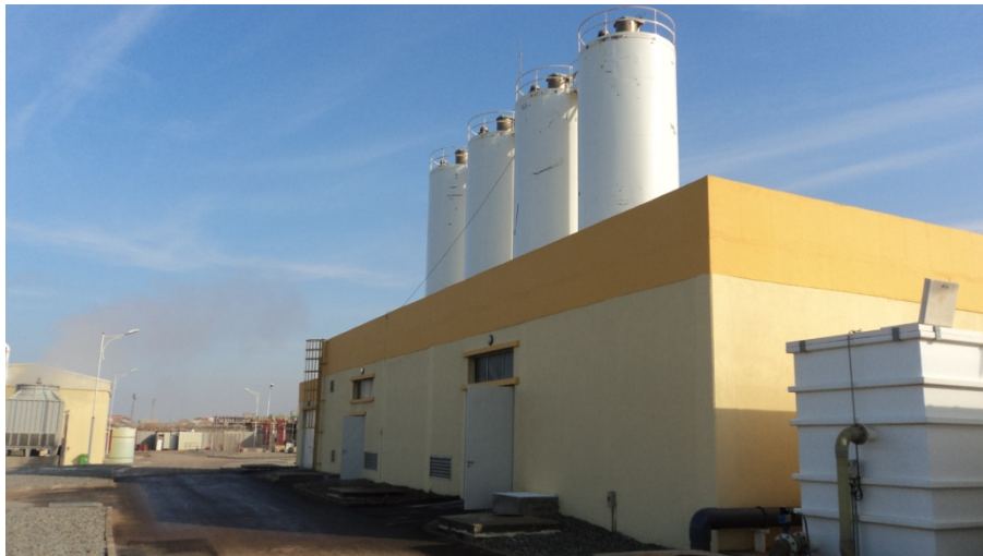
Figure V-12 : Silos de la chaux , [source: KHATEB.M].
