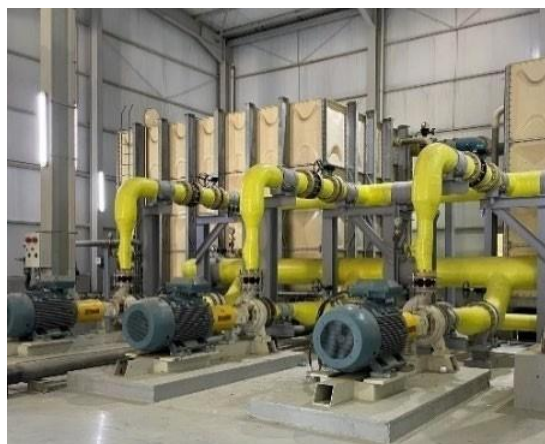
Figure 2.26. Pompes de nettoyage/ rinçage CIP
