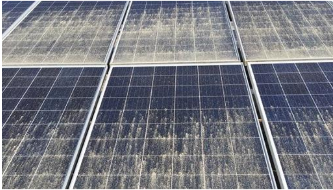
Figure 10: Effects of rain on solar panels [32].
