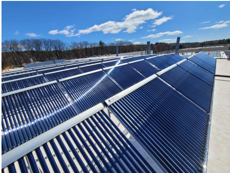
Figure 7: An image showing a field of thermal solar heat collectors.
