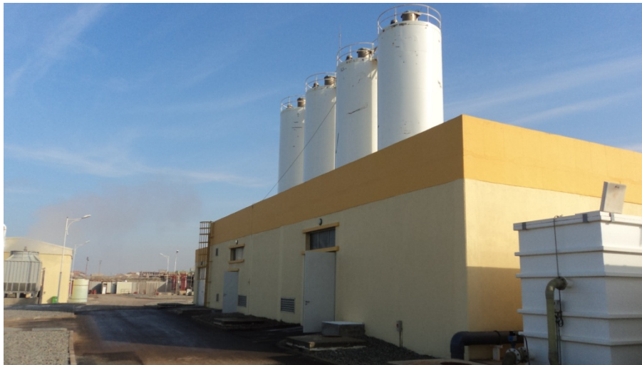
Figure V-12 : Silos de la chaux , [source: KHATEB.M].
