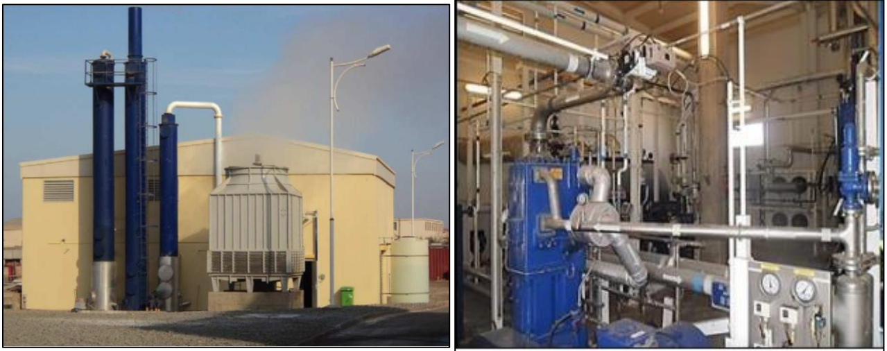
Figure II.26. Station de fabrication de CO 2 sur site.
