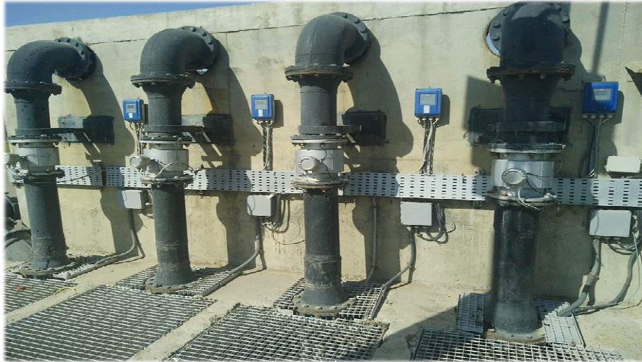
Figure 05 : Station de relevage.(Photo originale)
