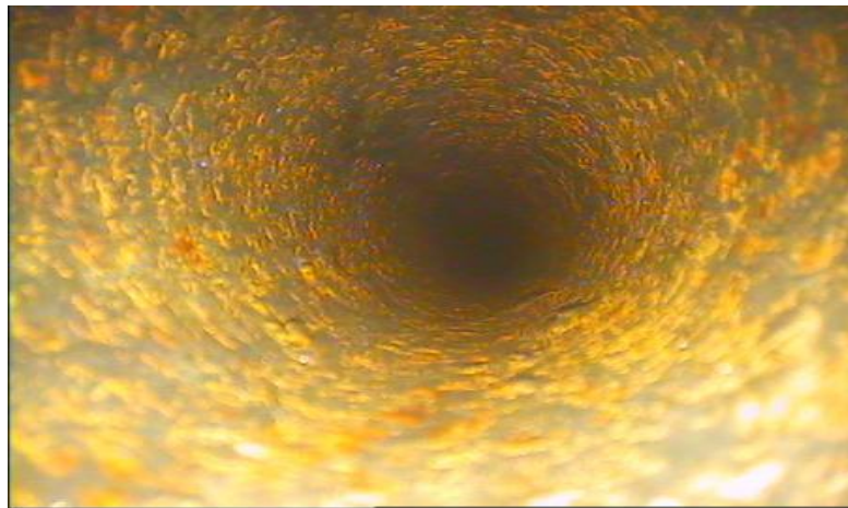
Figure 5.59: Corrosion interne de pipeline [10]
