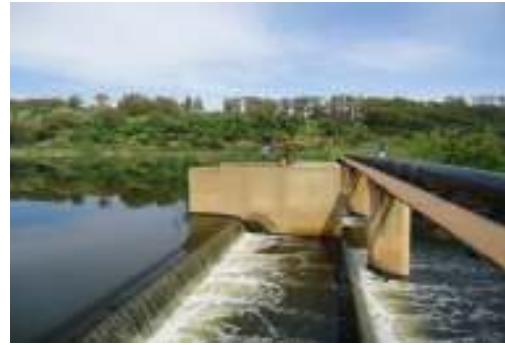
Figure 6 : station 1 (la digue)
