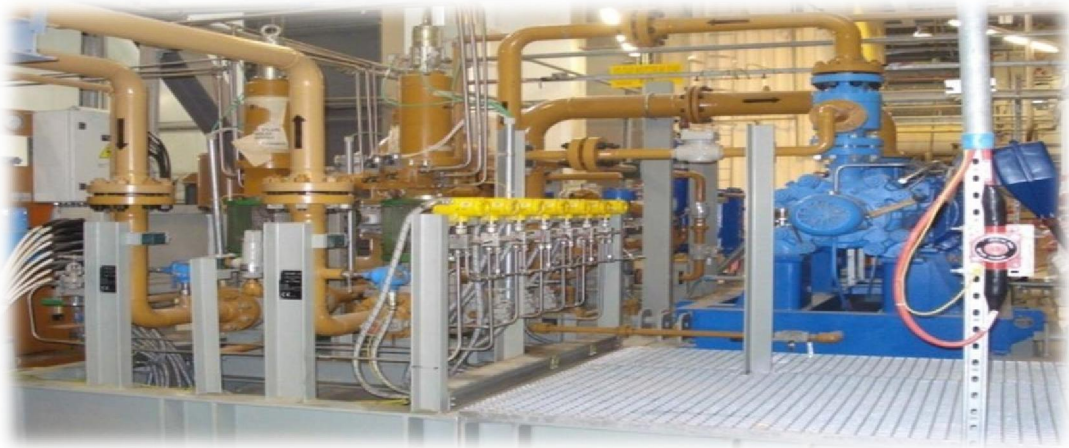
Figure I.14: station finale de fuel [6]
