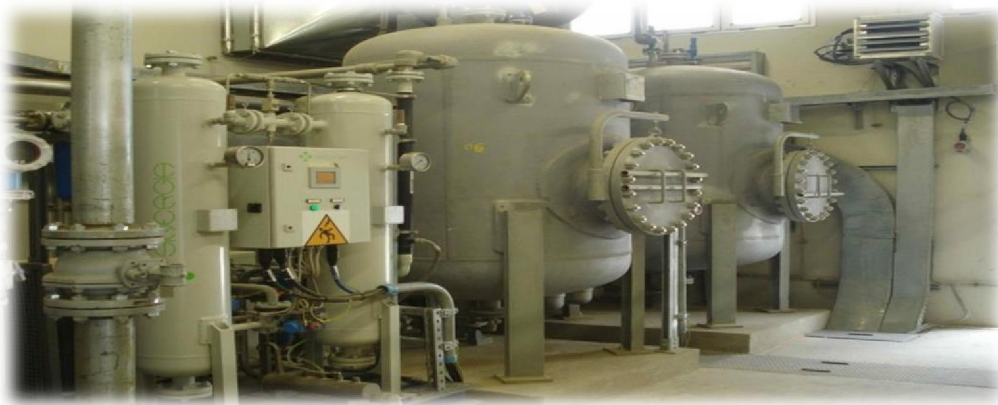
Figure I.12: station d l'air comprimé
