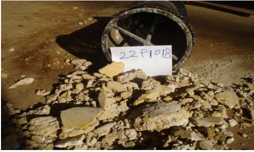
Figure II.2: bouchage de la pompe P-101B
