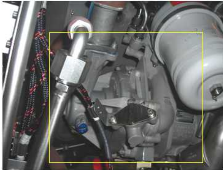
(Fig.III-2-1) pompe carburant.
