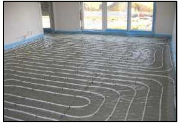
Figure 3-110: les planchers chauffants.
