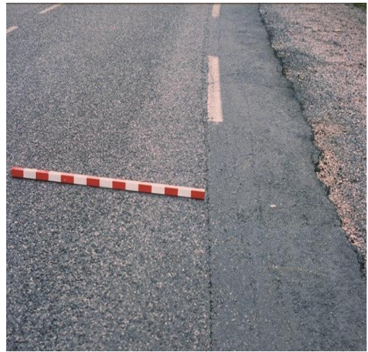
Figure 1.30 : Fissuration des joints [11].
