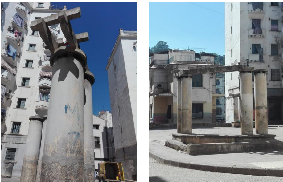
Figure 72 Parking ventilation pillars, cite Le Moulin between Colonel Lotfi Avenue and Ahmed Boudier Street Source: photographed by the author, 2020
