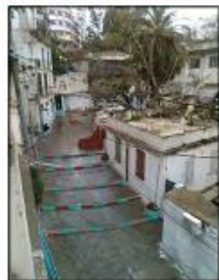
One floor buildings in a bad state along Houcine ROUBENH Street Source: Facebook page (Rampe Valée)
