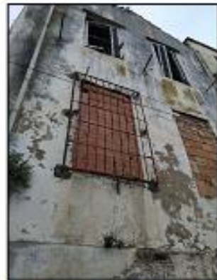
A 2 floors building in a very bad state along Houcine ROUBENH Street Source: Photographed by the author, 2020
