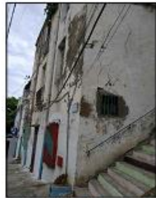
A 3 floors building in a bad state along Houcine ROUBENH Street Source: Photographed by the author, 2020
