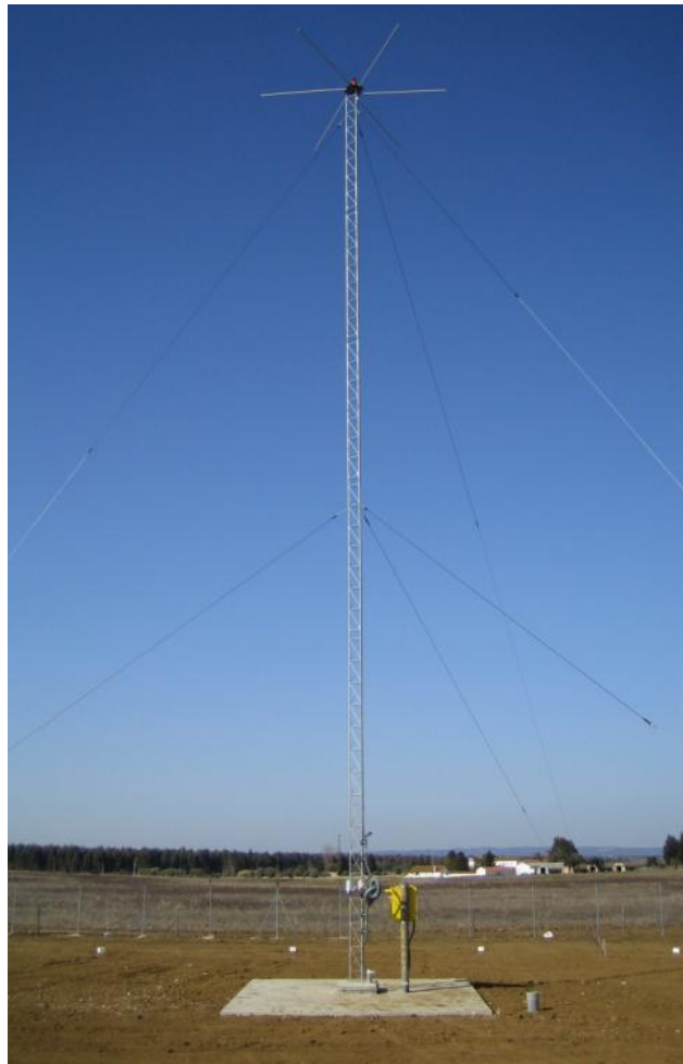
Figure III.1: Antenne d'une station NDB.
